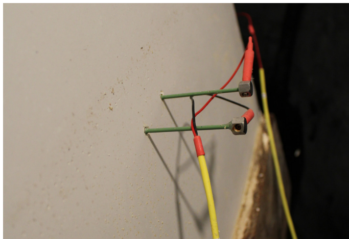
Figure 17 - Detail of Sample 2 assembly showing crystal granules formed on drywall after flooding
