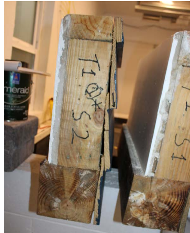
Appendix B4 Figure 12 - Sample 2 section view after the extended drying period.
