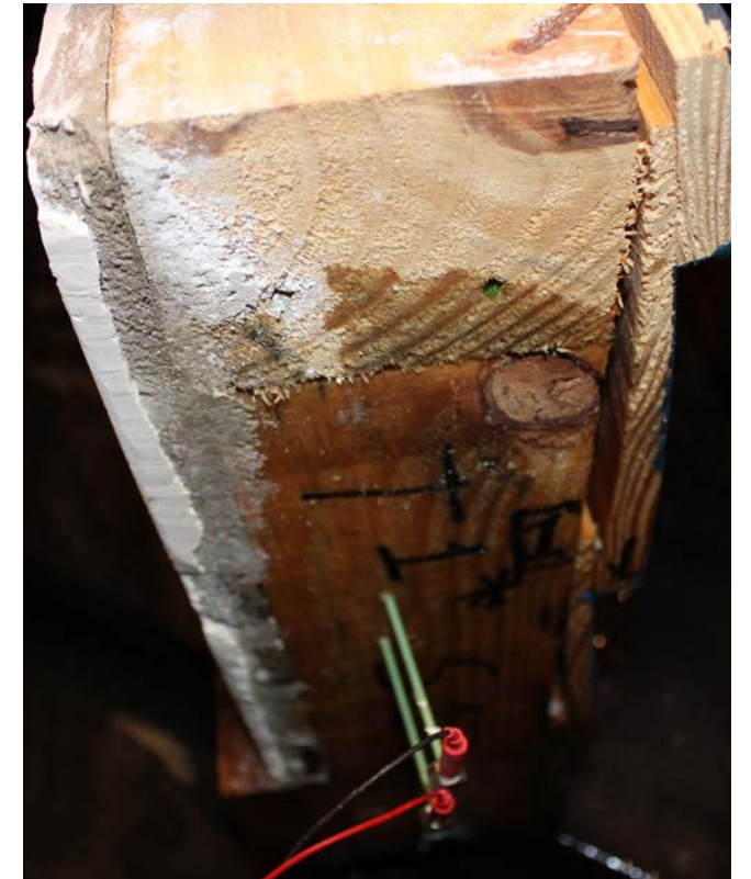
Appendix A3 Figure 14 - Sample 1 showing height of water absorption post-draining.
