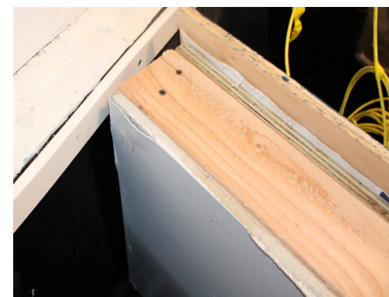
Wall Assembly 3 (drywall) peeling at edges post flooding
